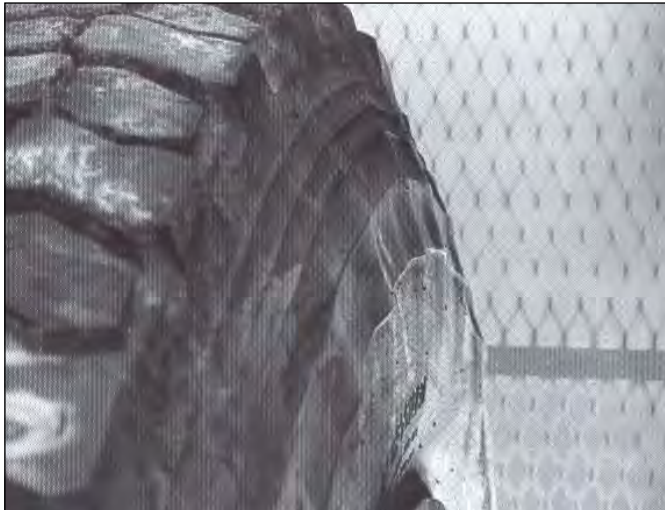
FIGURE 22: Using a grazing light or other indirect light source will produce shadows which indicate sidewall irregularities and/or signs of possible "zipper rupture."
