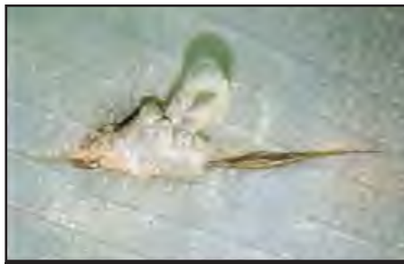
IMPROPER REPAIR (PLUG ONLY)
