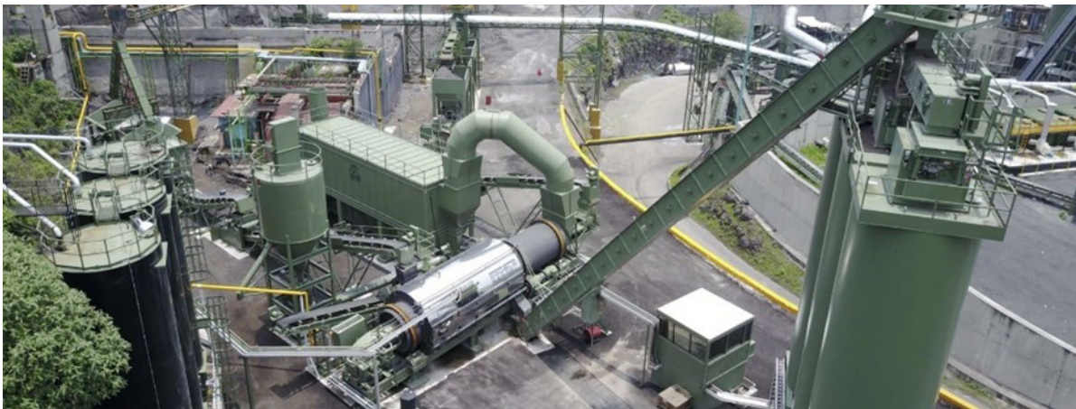
Figure 18. Asphalt plant are continuously evolving to capture emissions from being released to the atmosphere. Image from World Highways website.
