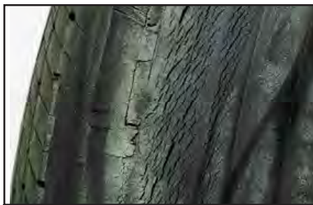
OZONE WEATHER CRACKING
